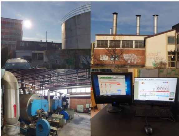
Figure 2. Building, boiler room and dispatcher centre in FMEDH
